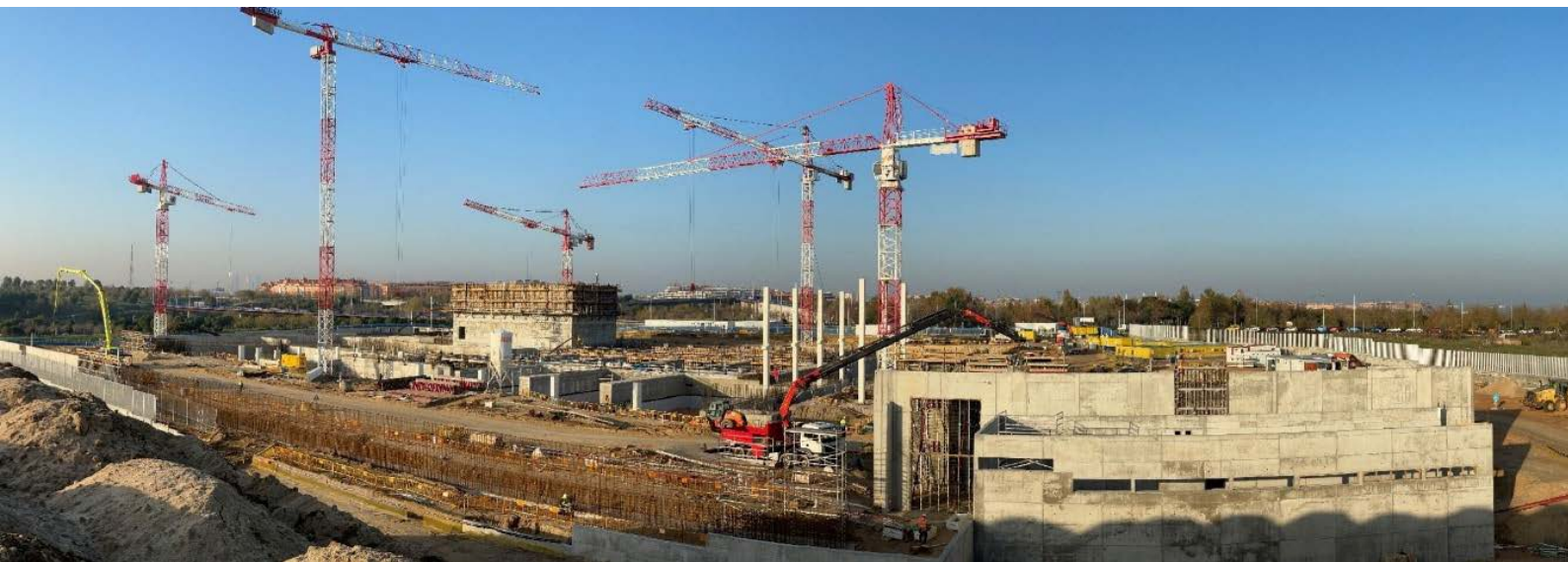
Construction of the new IMBISA facility commenced in March 2020 and is expected to finish in the fourth quarter of 2021.
